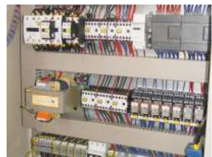
Switching cabinet / SPS control
